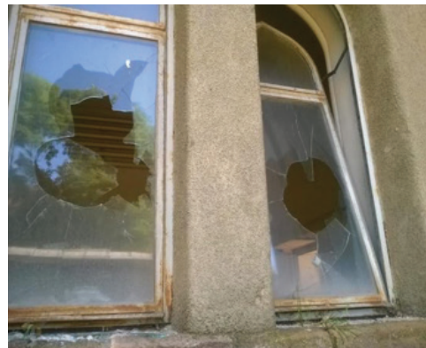
The broken windows of the Synagogue in Gyöngyös,
