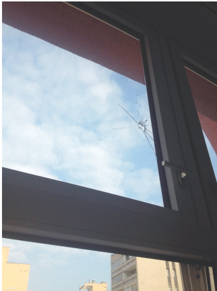
A window broken with ball bearings. Source: Index
